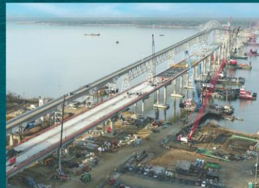
Skanska -Corman-McLean brought together the largest construction marine fleet in the East Coast to concurrently build 200-ft long deep foundations; 135-ft tall piers; 95” deep and 175-ft long concrete girder spans; and 12-ft deep and 350-ft long steel spans.
