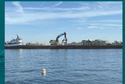
Sustainability at its Best: Using recycled concrete from the demolition of the original bridge, artificial reefs were built to create fish habitat.
