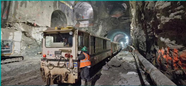
Station cavern excavation. Situated approximately 140-feet below Park Avenue, one of the two approximately 1,200-foot-long, three-level caverns that were created using tunnel boring machines, road headers and drill-blast excavations. Completion required more than 3,000 blasts.
