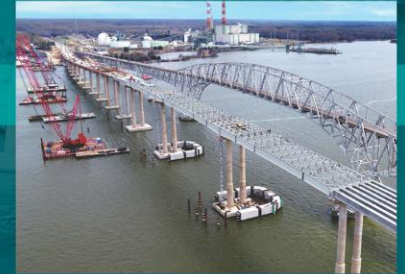
Designed and permitted in 11 months, construction started four months early in 2020 and continued during the COVID-19 pandemic.
